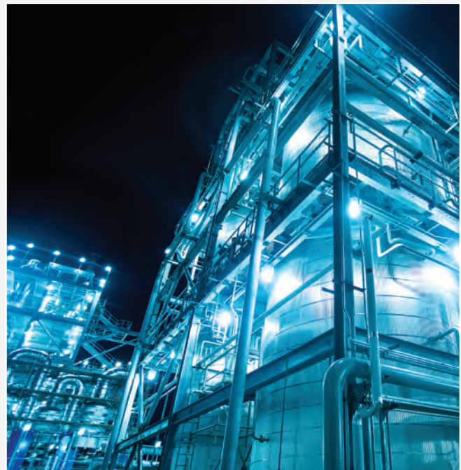
Myriant's Lake Providence Commercial Facility for Bio-Succinic Acid
